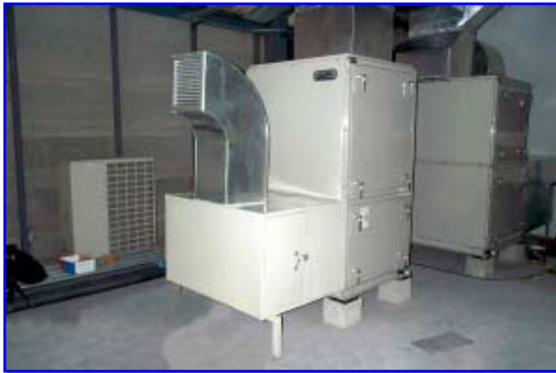
Standalone fresh air unit on outdoor installation using DX coil with wrap around Heat Pipe
