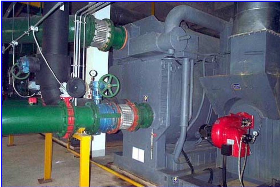
Direct fired absorption chiller installation in China.
