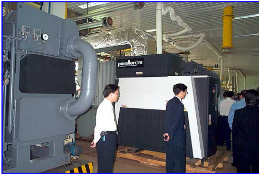
Small gas turbine coupled with Direct exhaust absorption chiller.
