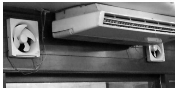
Fig. 8. Under ceiling unit installation with exhaust fa
