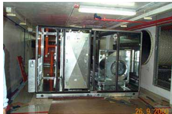
Figure 14. Outdoor air unit with wrap around heat pipe that supply dry fresh air into the building
