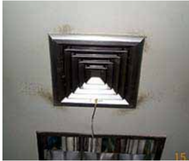
Figure 1. Dirty ceiling supply air diffuser which normally found in infiltrated building
